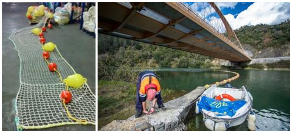
Figure 10 : Barrier (left) installed in Deba river (right)
